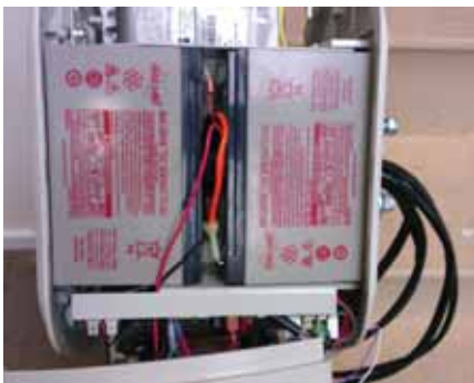
BATTERIES ROTATED BACK IN PLACE
