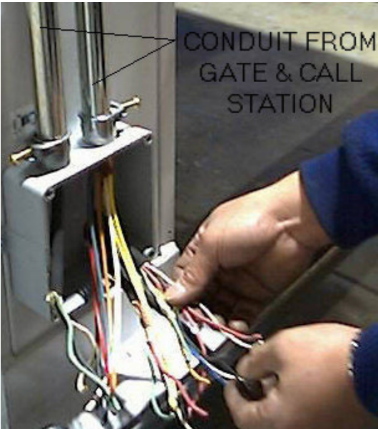
FIG. 18- WIRING OUTSIDE JUNCTION BOX
